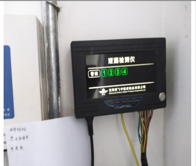
输油管线渗漏检测
